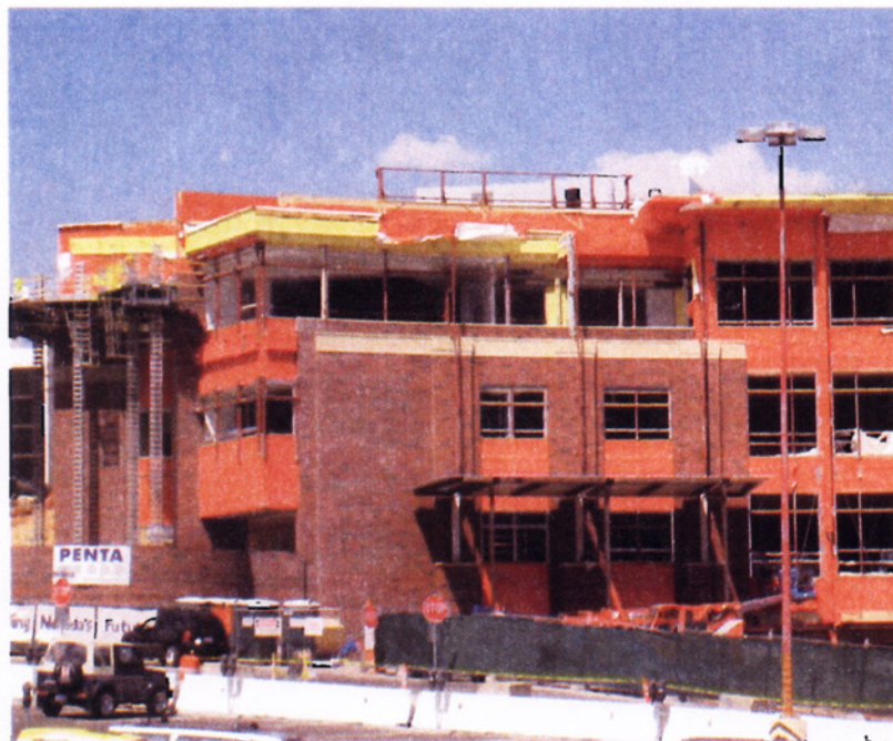
A steeply sloping and tight construction site along with the neighboring construction at the Knowledge Center made logistics a challenge.
